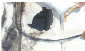
Deterioration over time
